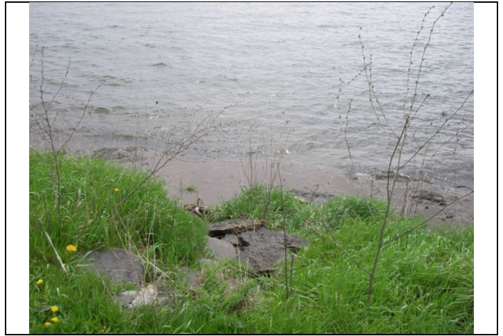
Photo 2 Station 10 – downstream view from South Shore Road, perched culvert outletting to limestone bedrock along Lake Ontario shoreline
