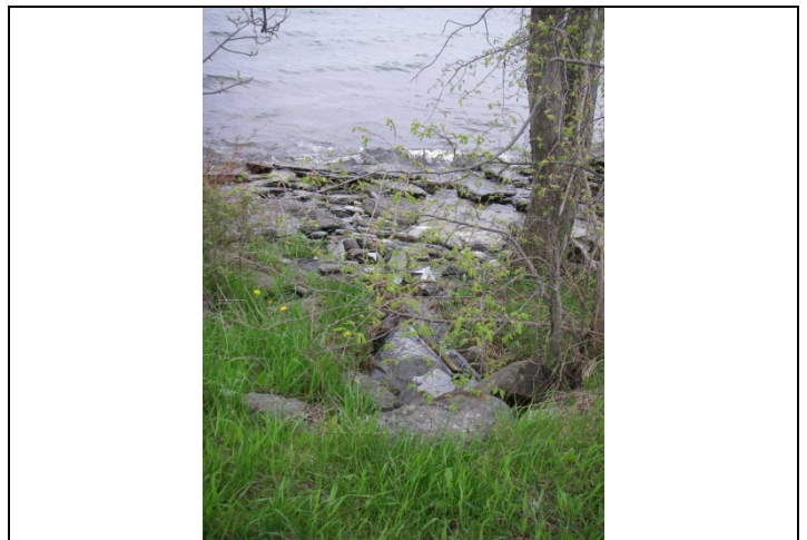
Photo 6 Station 13 – downstream view from South Shore Road, perched culvert outletting to limestone bedrock along Lake Ontario shoreline
