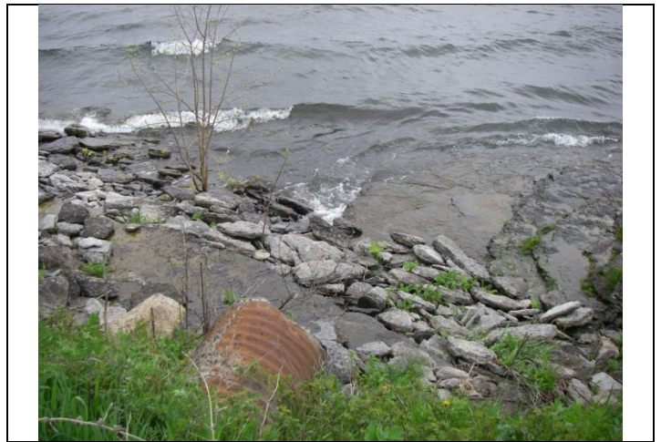
Photo 4 Station 12 – downstream view from South Shore Road, perched culvert outletting to limestone bedrock along Lake Ontario shoreline
