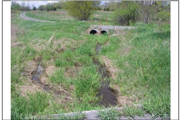
Photo 2 Station 30 – downstream view of braided flow through grasses situated between Front Road and driveway access road
