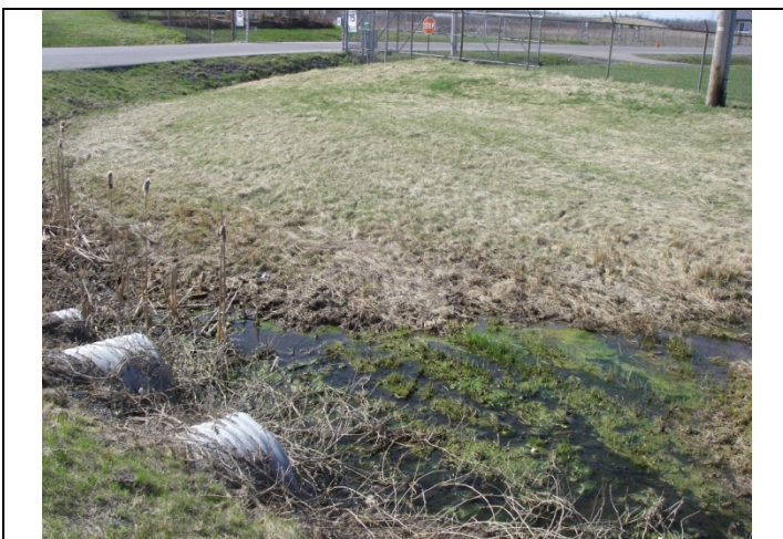
Photo 9 M4 – Facing upstream from Taylor Kidd Boulevard showing lack of channel.
